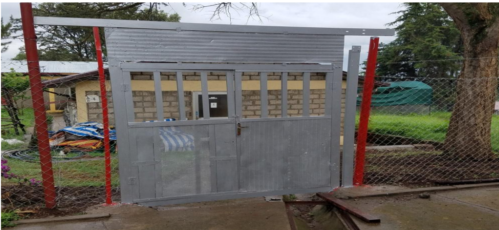
Fig.34. Greenhouse and growth chamber compound fenced, door and different parts of growth chamber houses constructed and furnished
